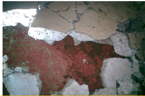
Burst concrete pipe due to pressure transfer
