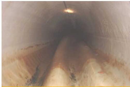
Lumps caused by ground water pressure
